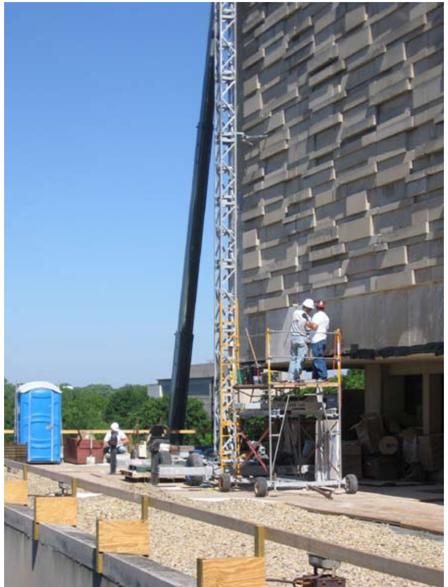
Construction on the Wells Library to repair the distinctive building's patterned limestone siding.
